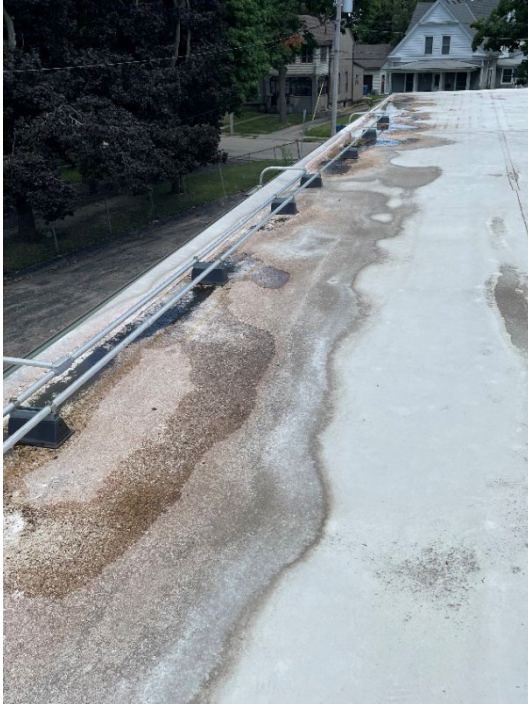
Photo #PC5 – Additional ponding near edge of roof
