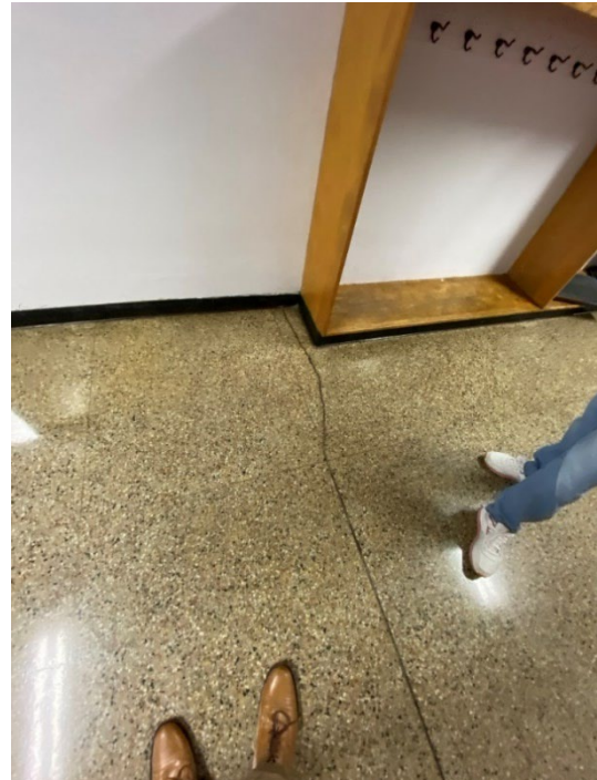
Photo #HF4 – Floor crack
