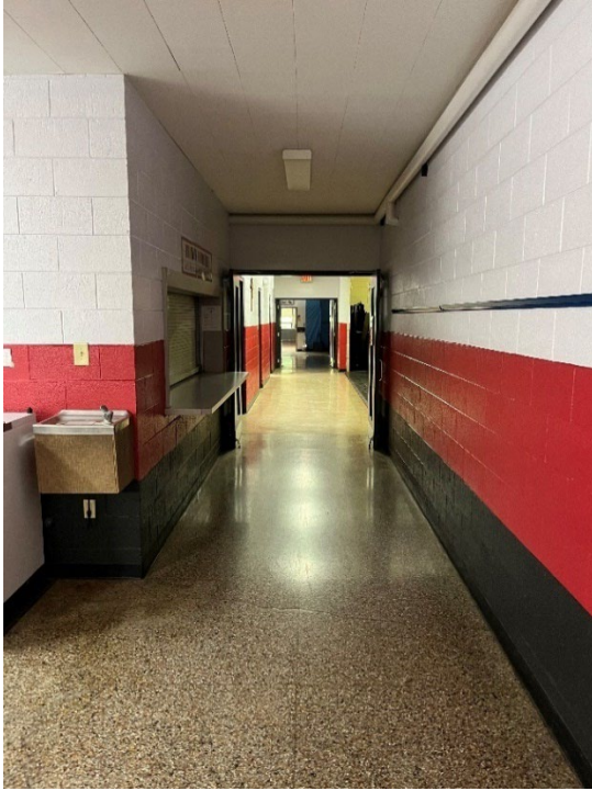
Photos – #HF9– Protruding counter
