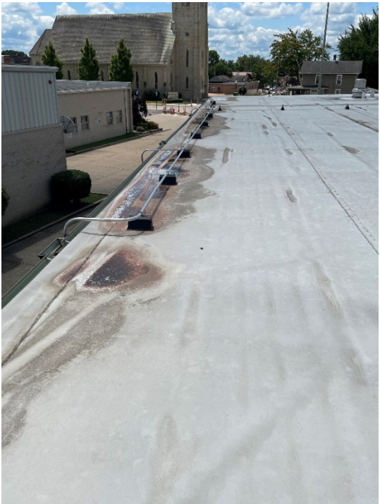
Photo #PC4 – Ponding near edge of roof
