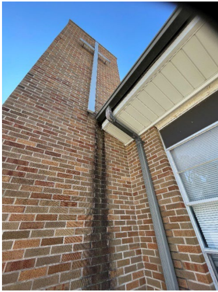
Photo #TC1 – Staining at gutter termination
