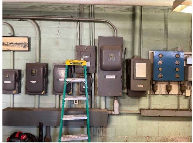
Photo #TC6 – Distribution of electrical panels using six disconnect rule
