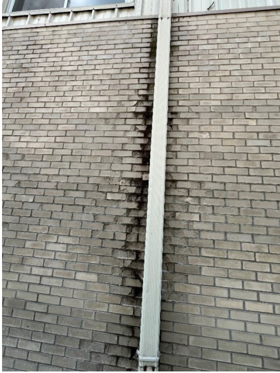
Photo #PC2 – Spalling behind downspout on gymnasium addition
