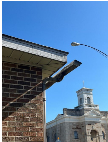
Photo #TC2 – Gutter pulled away from roof edge
