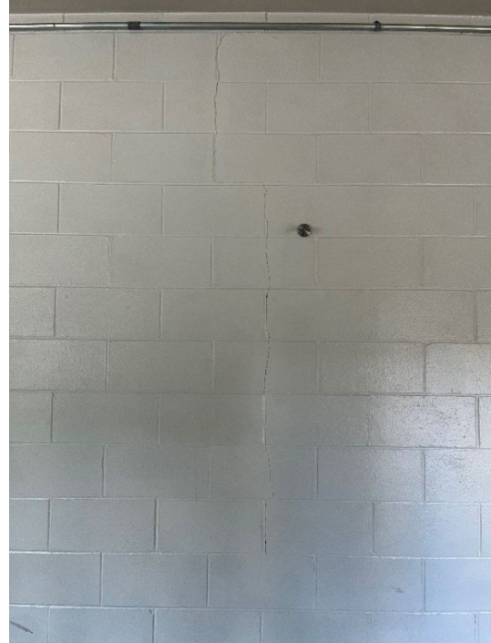
Photo - #PC6 – Crack in Corridor to Gym Addition
