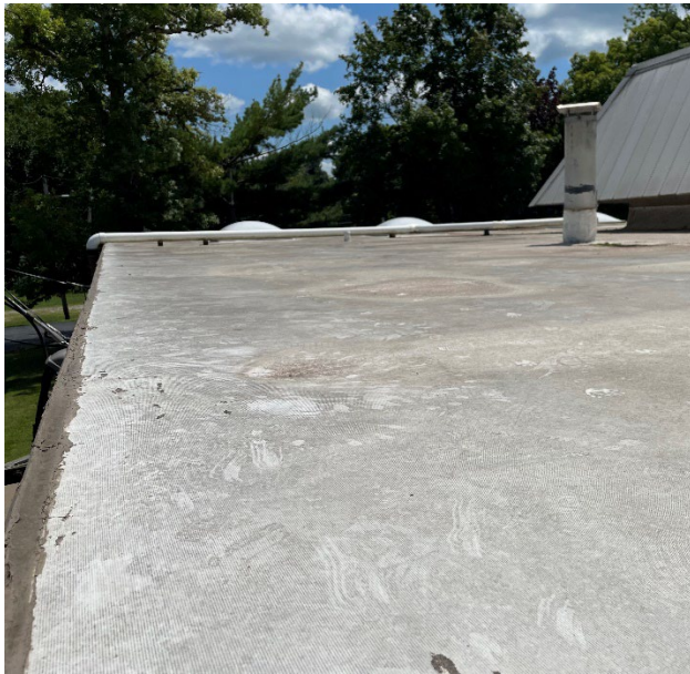
Photo #HF3 – Evidence of ponding on low roof
