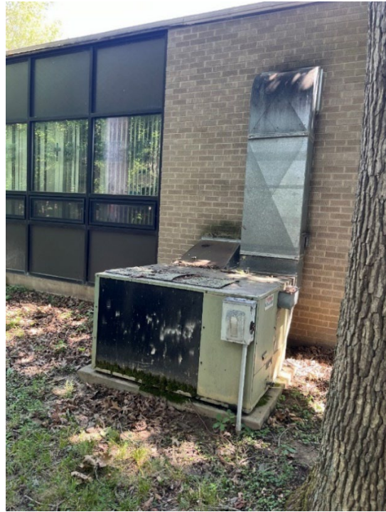
Photo #HF6– Weathered AHU (northwest)
