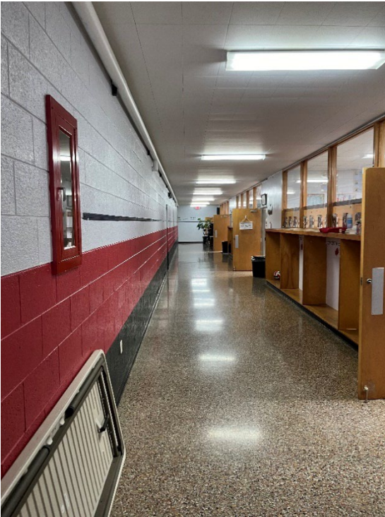
Photo #HF7 – Non-rated corridor condition
