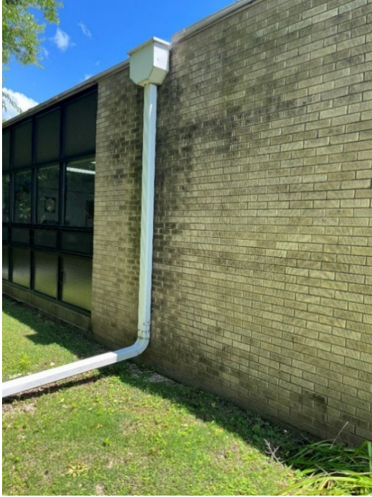
Photo #HF1 – Staining and potential infiltration at conductor & downspout.
