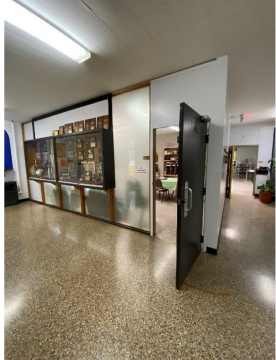
Photo #HF8 – Non-rated corridor condition
