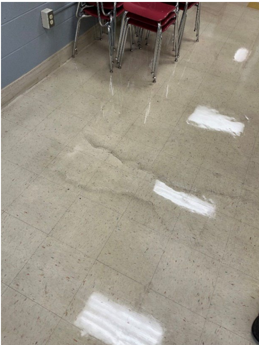
Photo - #PC7 – Heaved Floor Slab at Lower Level
