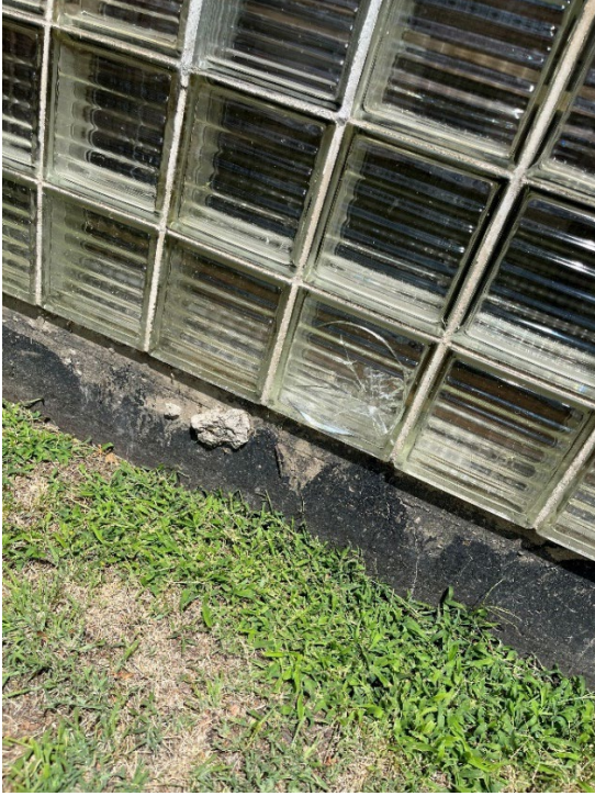
Photo - #PC1 – Fractured Glass Block Unit near Entrance
